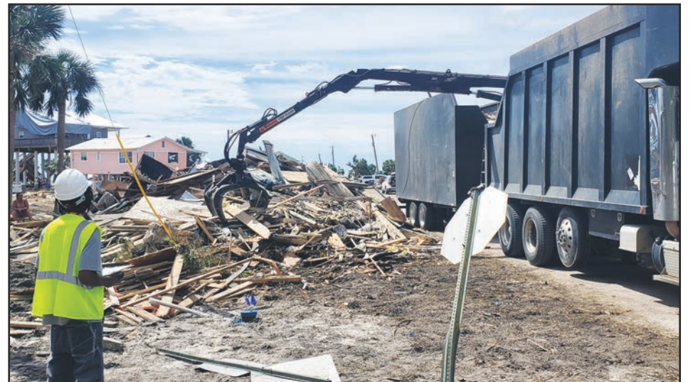
Some 42 debris removal trucks -- contracted with through the FDOT -- are busy working all around the county hauling away downed trees and the splintered remains of homes at Dekle Beach (above) and other coastal areas destroyed by Hurricane Helene.
